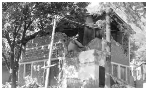
Figure 6.1 : A Damaged Building Due to an Earthquake
